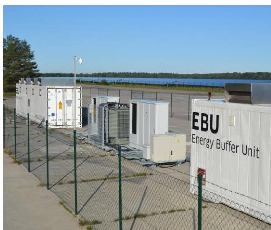
Photo: BELECTRIC EBU at the solar power plant Alt Daber, Germany
