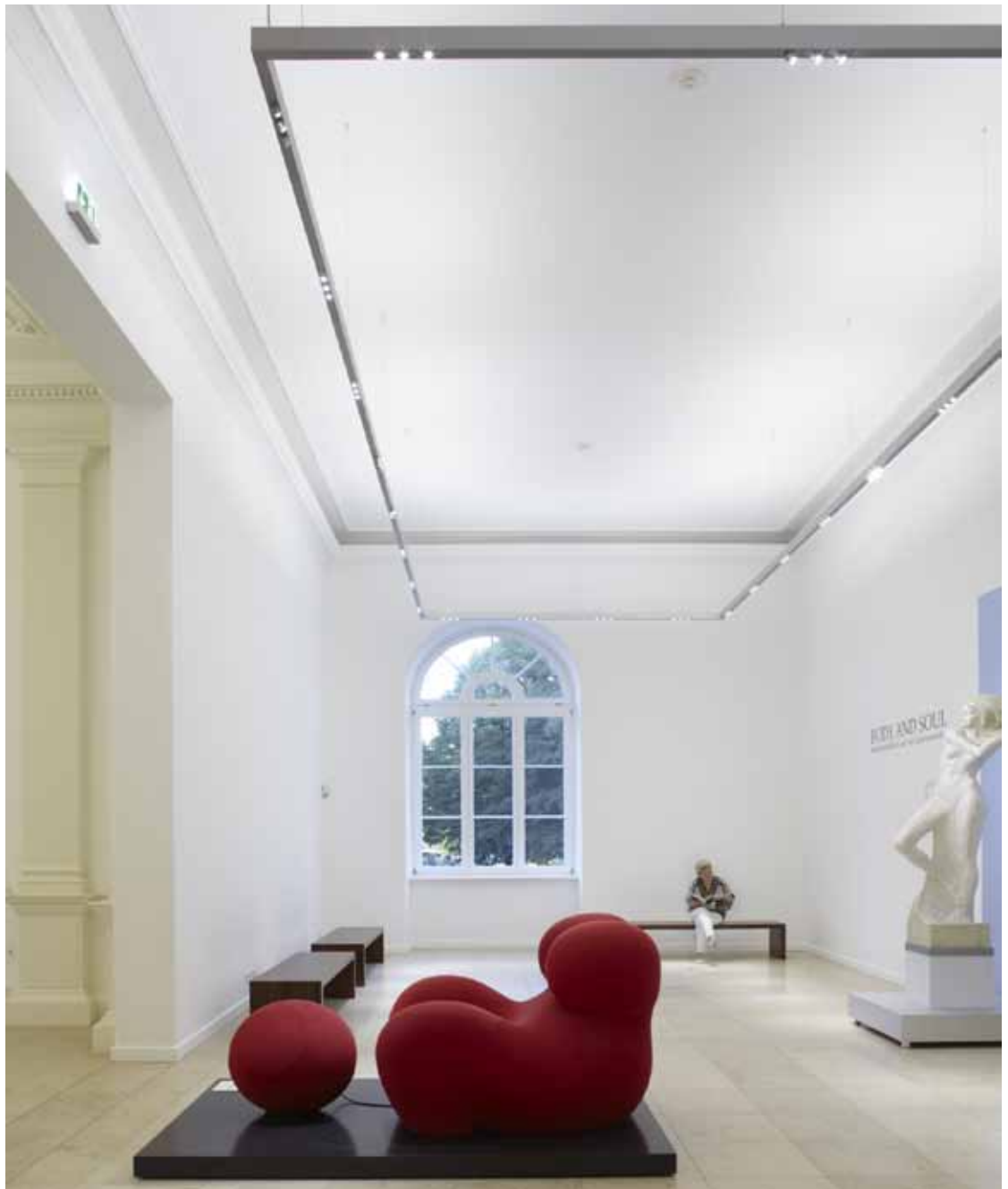
B5 | The Supersystem aluminium trunking system inconspicuously blends into the architecture, its UV- and IR-free light ensuring gentle illumination of the exhibits.
